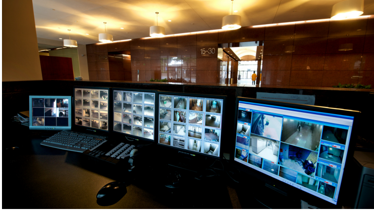
Security Monitoring System
